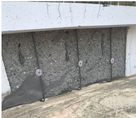
Fig. 15. Beam 4 after injection of shear cracks, concrete hammering, sandblasting, drilling of the holes in the flange, installation of the U-shaped ribbed memory-steel stirrups. The strengthening steps 5 to 9 are still missing in the photo.
