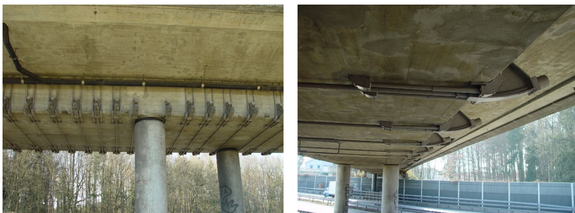
Fig. 1. Example of a conventional shear strengthening on a Bridge near Solothurn in Switzerland.
