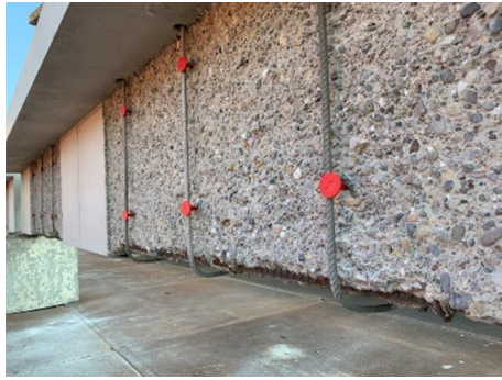
Fig. 3. Installed memory-steel stirrups on one of the test beams. The red bolts are polymer dowels for fixation of the memory-steel stirrups on the concrete surface. (For interpretation of the references to colour in this figure legend, the reader is referred to the web version of this article.)
