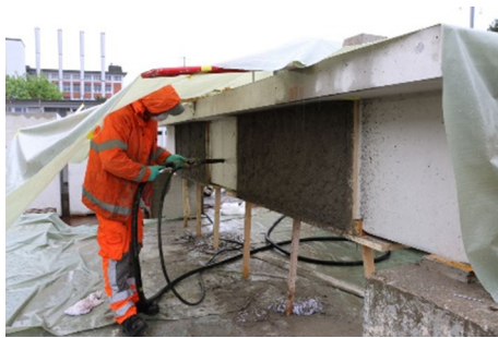
Fig. 4. Application of spray mortar to one of the test beams. Timber formwork on the sides and the bottom.
