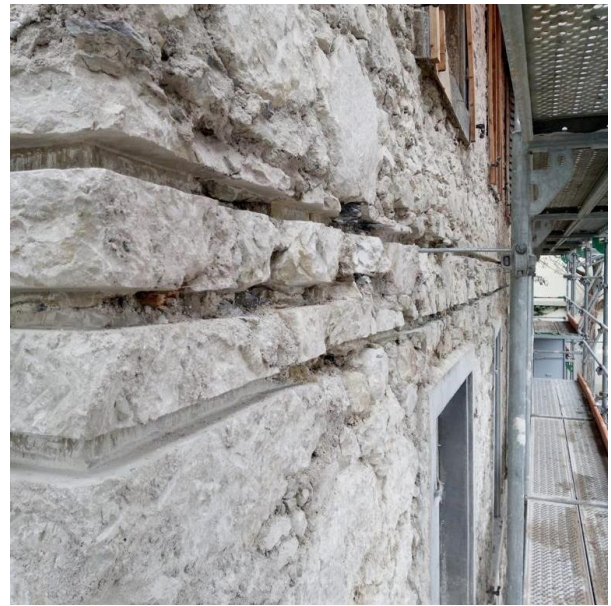
Grooves in rubble stone masonry
