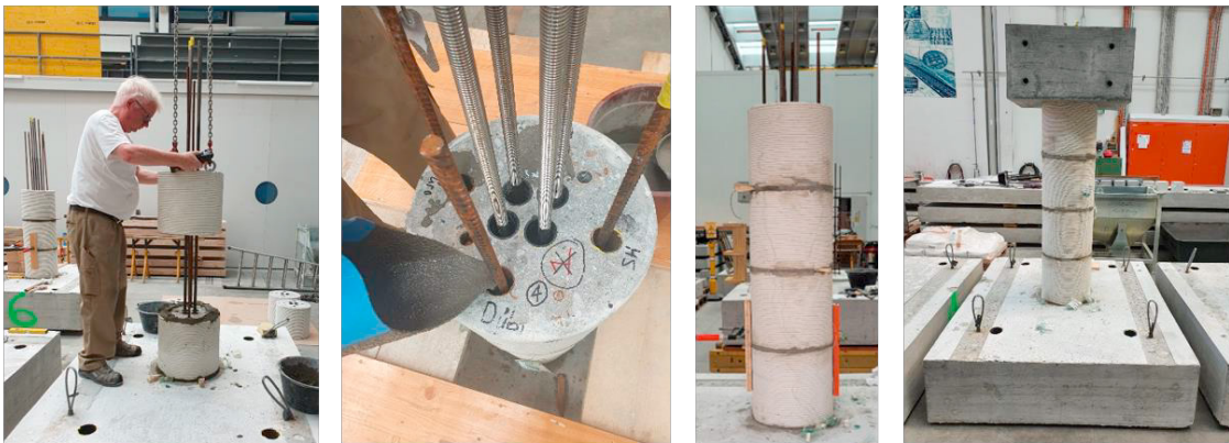
(e) Stacking of segments (f) Grouting of reinforcement (g) Assembled column segments (h) Completed column assembly
