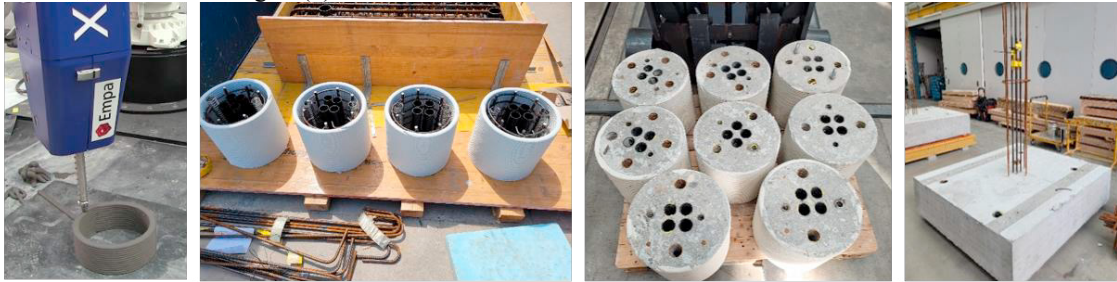
(a) 3D printing of formwork (b) Installation of reinforcement and ducts (c) Cast concrete filling (d) Cast footing with reinforcement
